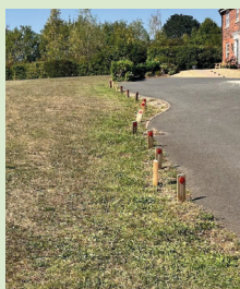
Before - broken and missing bollards
